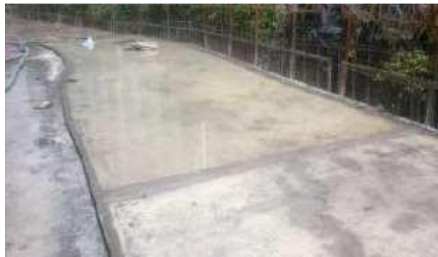
Fig:16 Ponding of slab
